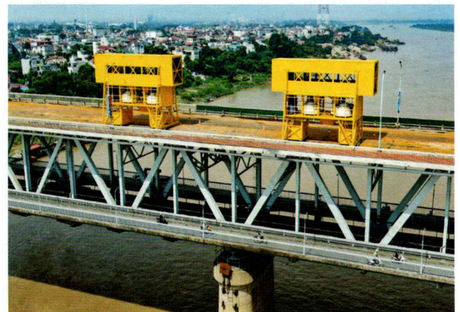
Application of mobile ultra-high-performance concrete (UHPC) batching plant in Thang Long bridge deck repair.
