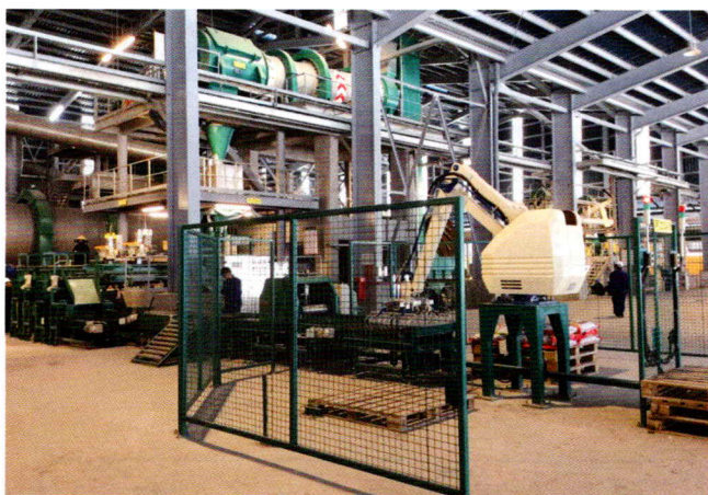
Automatic NPK bagging transportation system
